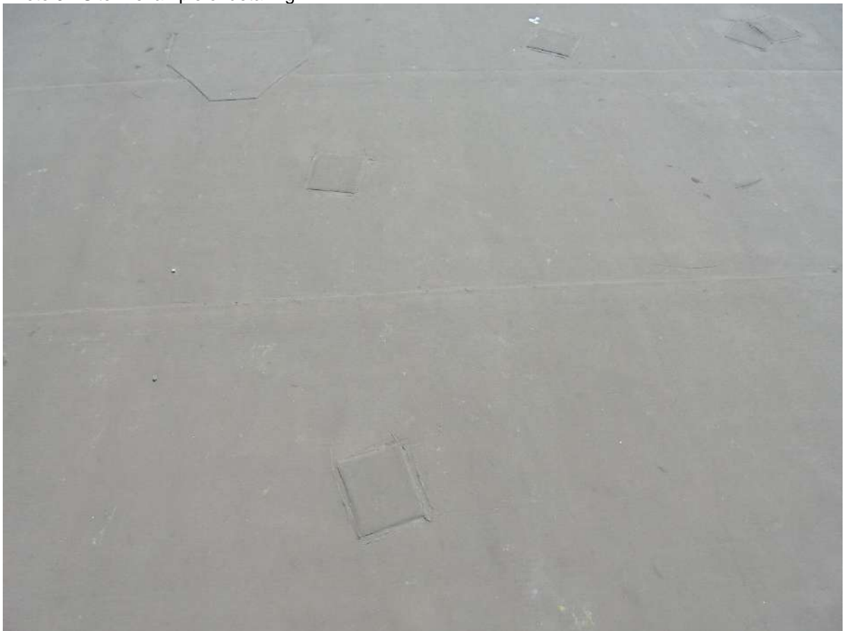
Photo 4 - Site A example of patch repairs
