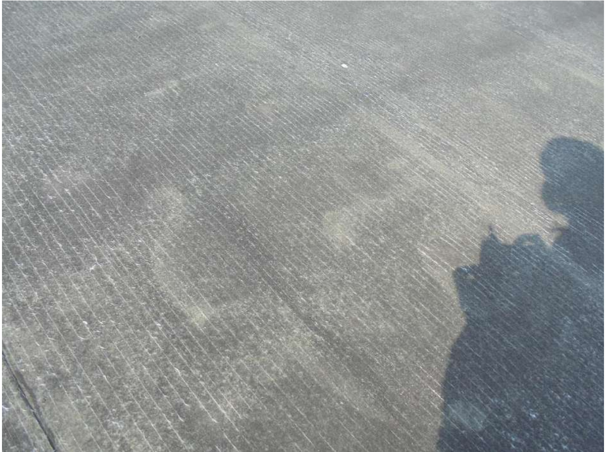
Photo 3 – Top glass reinforcement visible
