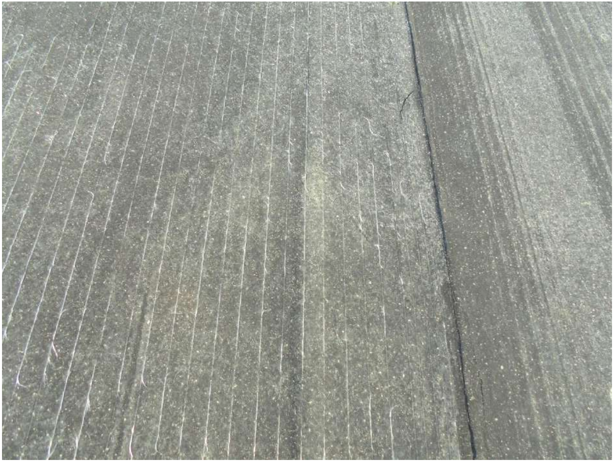
Photo 3 –Site C broken strands of glass reinforcement
