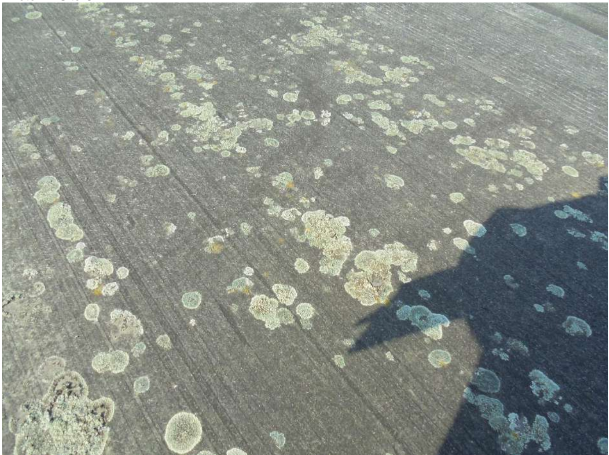
Photo 2 - Site C example of lichen growing on the membrane
